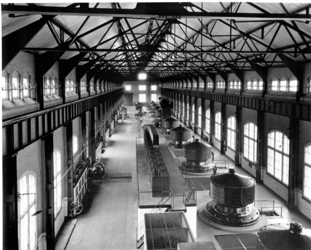
Niagara Falls Station
